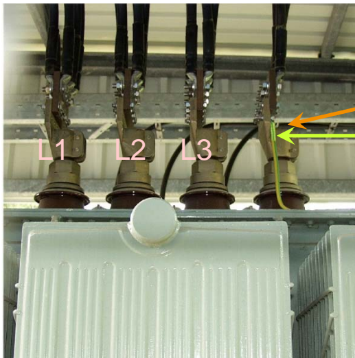
Transformer at DESY
